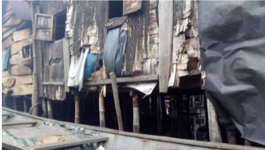
Plate 4. A typical building wall condition in Makoko (Source: Authors' fieldwork, 2016).
