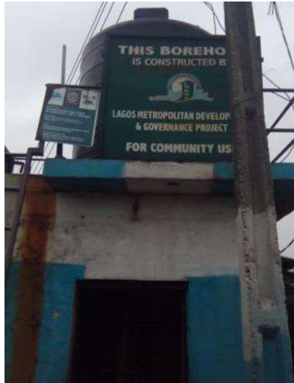
Plate 8. A dilapidated borehole tank (Source: Authors' fieldwork, 2016).
